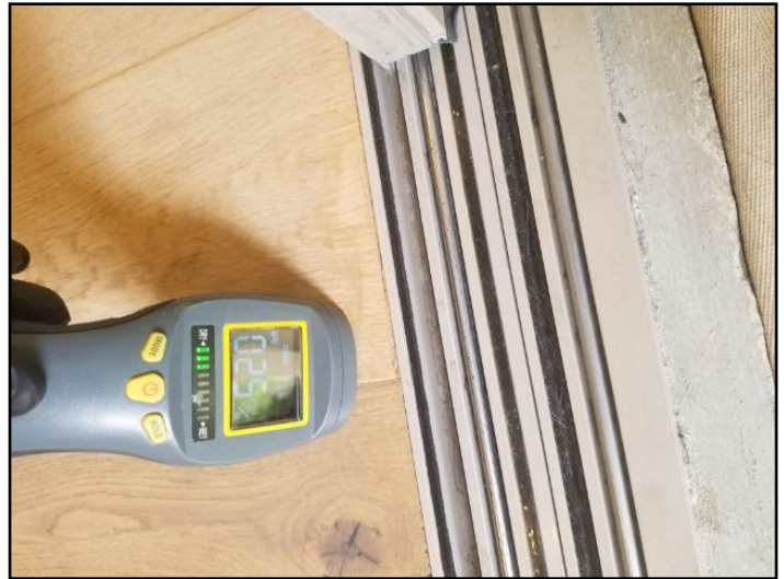
26. Damaged, cracked or loose
