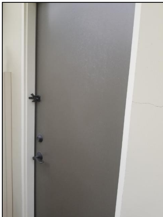
65. Damaged, cracked or loose
