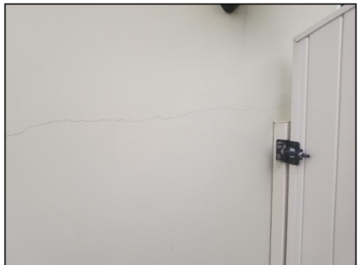
64. Damaged, cracked or loose
