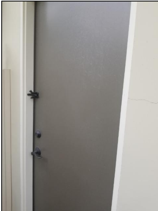
25. Damaged, cracked or loose
